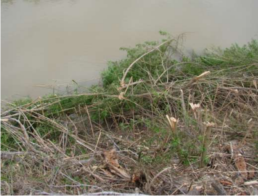
More bank damage.
